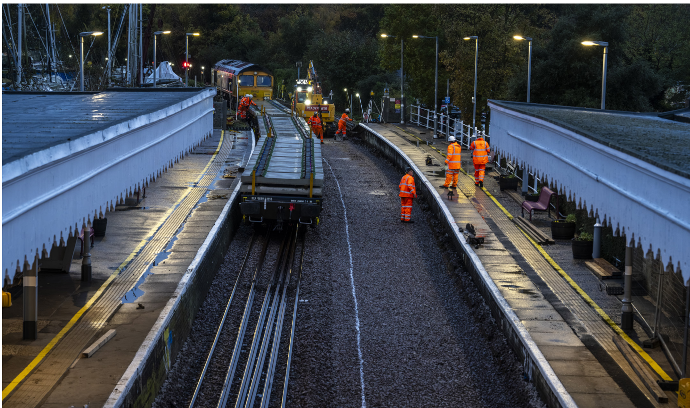
Track renewal project in a station. Image Credit South Rail Systems Alliance (SRSA)
