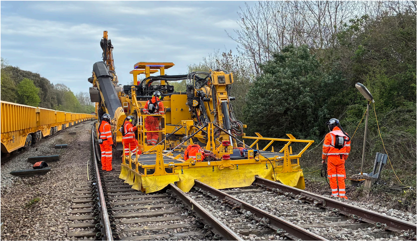
A typical track renewal project being delivered. Image Credit South Rail Systems Alliance (SRSA)
